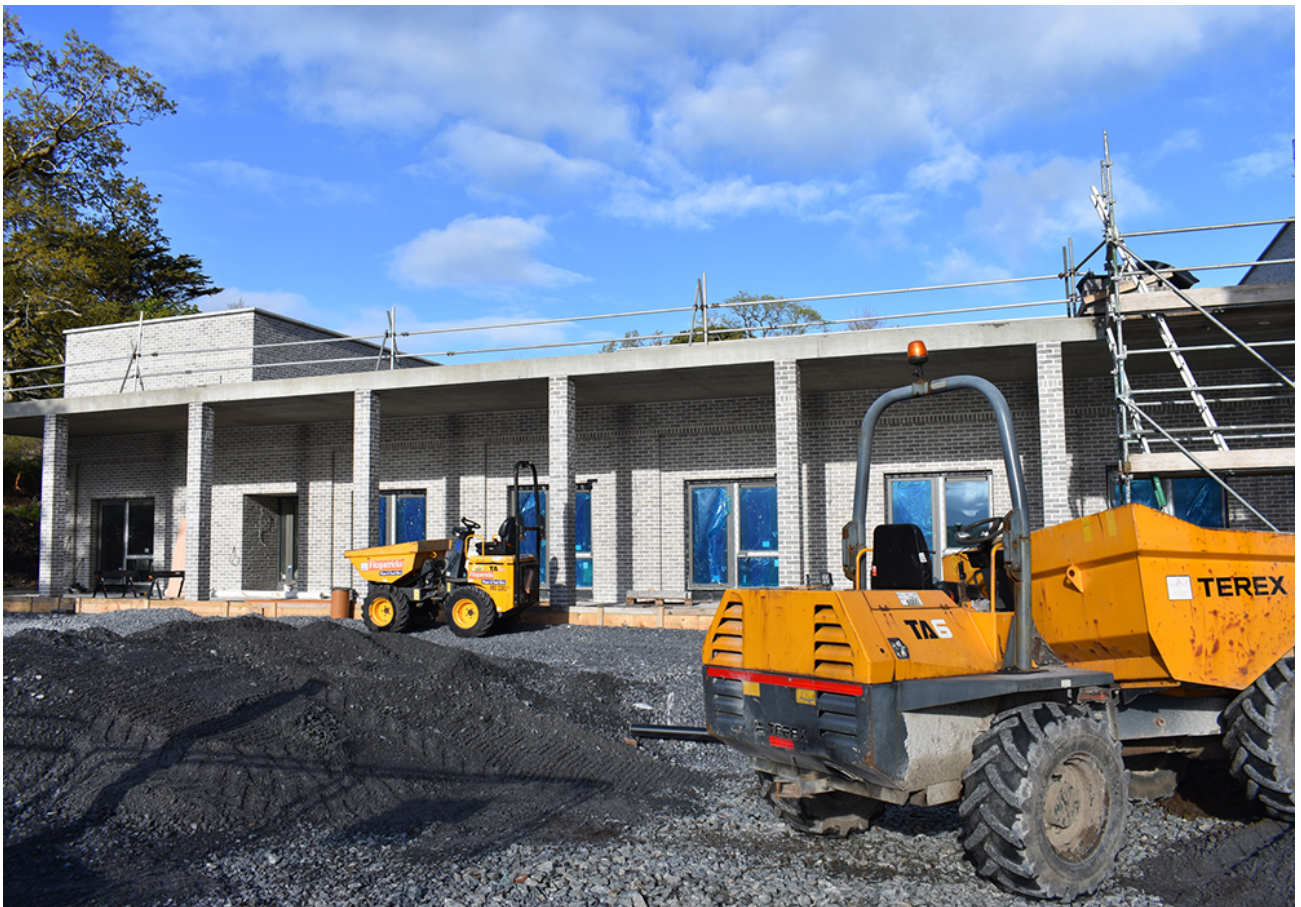
Equipment is visible on what will be the public side of the new monastery at Kylemore Abbey in the final weeks of construction. (Julie A. Ferraro)
