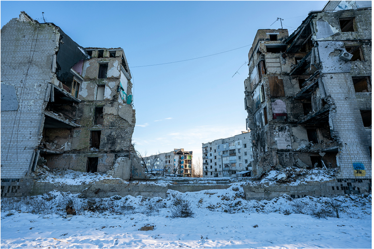
The center of this apartment complex in Borodyanka, Ukraine, collapsed when a Russian missile hit it on April 5, 2022. (Gregg Brekke)
