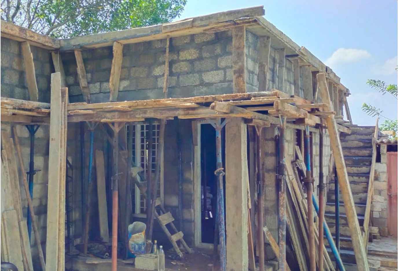
The walls of the new house under construction (Courtesy of Rose Cherian Vachaparampil)
