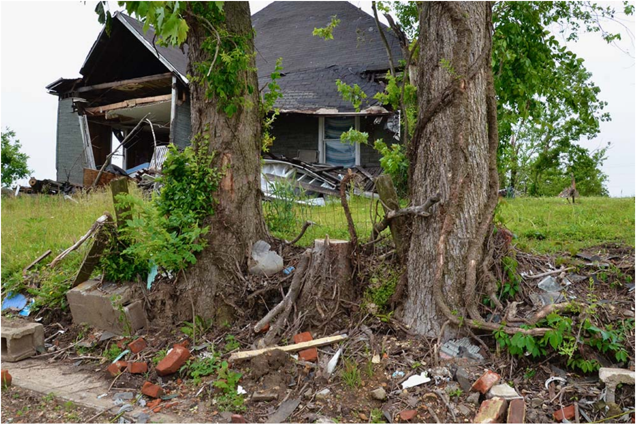
A home damaged by a Dec. 10 tornado awaits demolition May 23 in Mayfield, Kentucky. (GSR photo/Dan Stockman)
