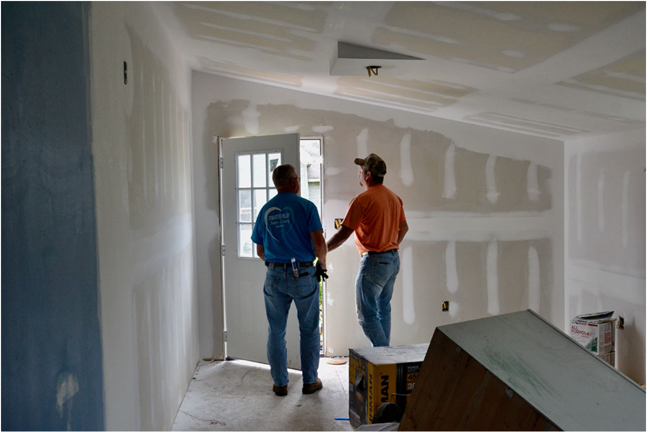
David White, left, and Ronnie Mattingly check out a leaky door May 23 at a house in Mayfield, Kentucky, damaged by a tornado in December. (GSR photo/Dan Stockman)
