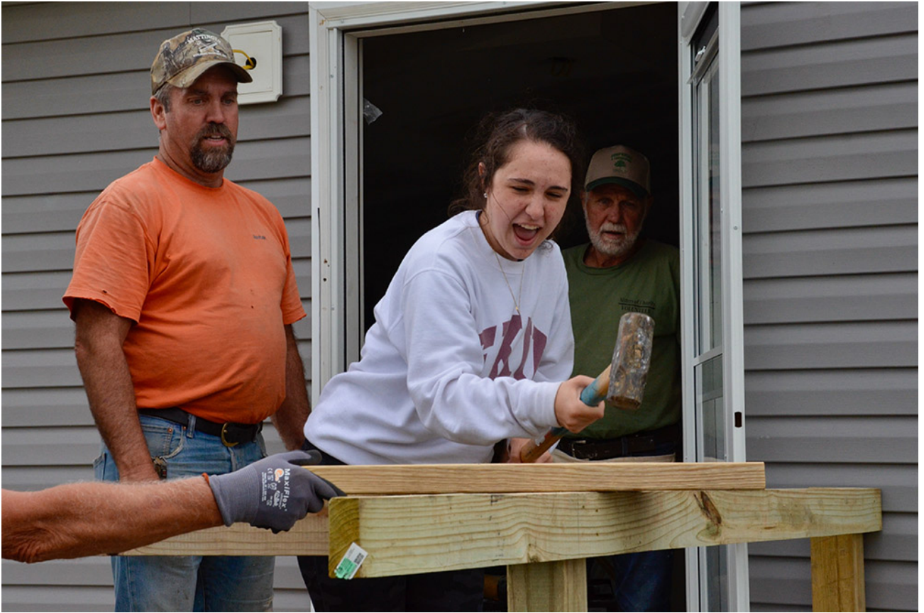
Ronnie Mattingly, left, and Jude Leake watch Lizzi Seyle try the sledgehammer May 23 as the disaster recovery team works on a home damaged by a Dec. 10 tornado in Mayfield, Kentucky. (GSR photo/Dan Stockman)
