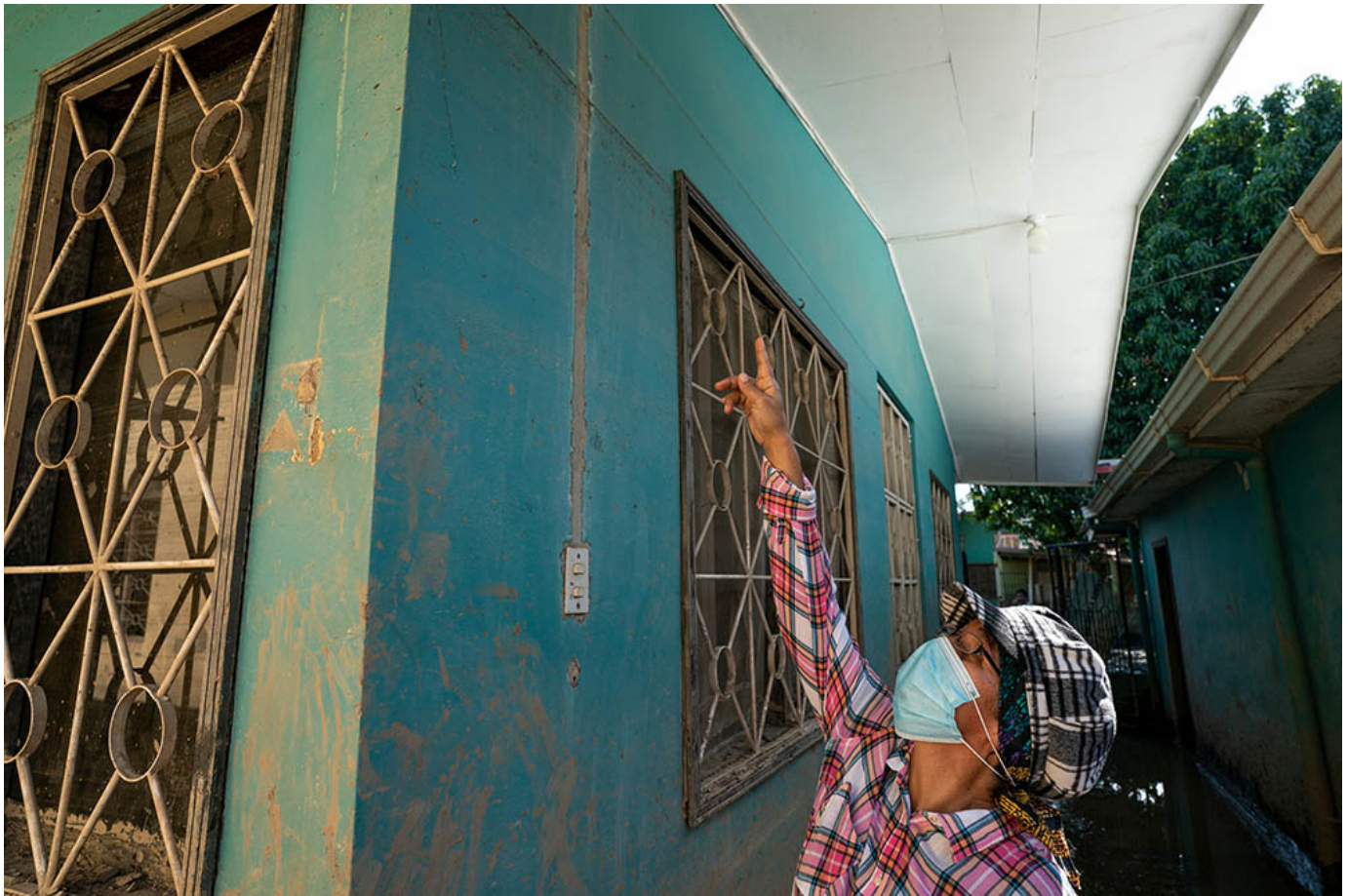
Sr. Victoria Emérita points to the floodwater line on a building at Our Lady of the Holy Fountain Nursery School in La Lima, Honduras. (Gregg Brekke)
