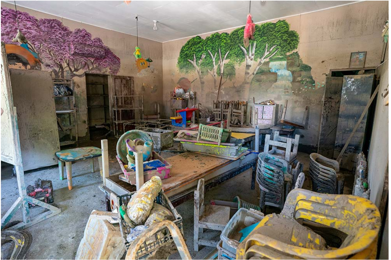
A flood-damaged classroom at Our Lady of the Holy Fountain Nursery School (Gregg Brekke)
