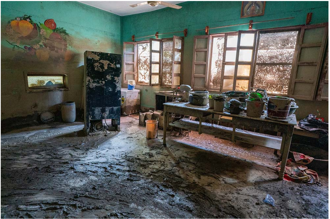
The dining area at Our Lady of the Holy Fountain Nursery School, damaged during Hurricanes Eta and Iota (Gregg Brekke)
