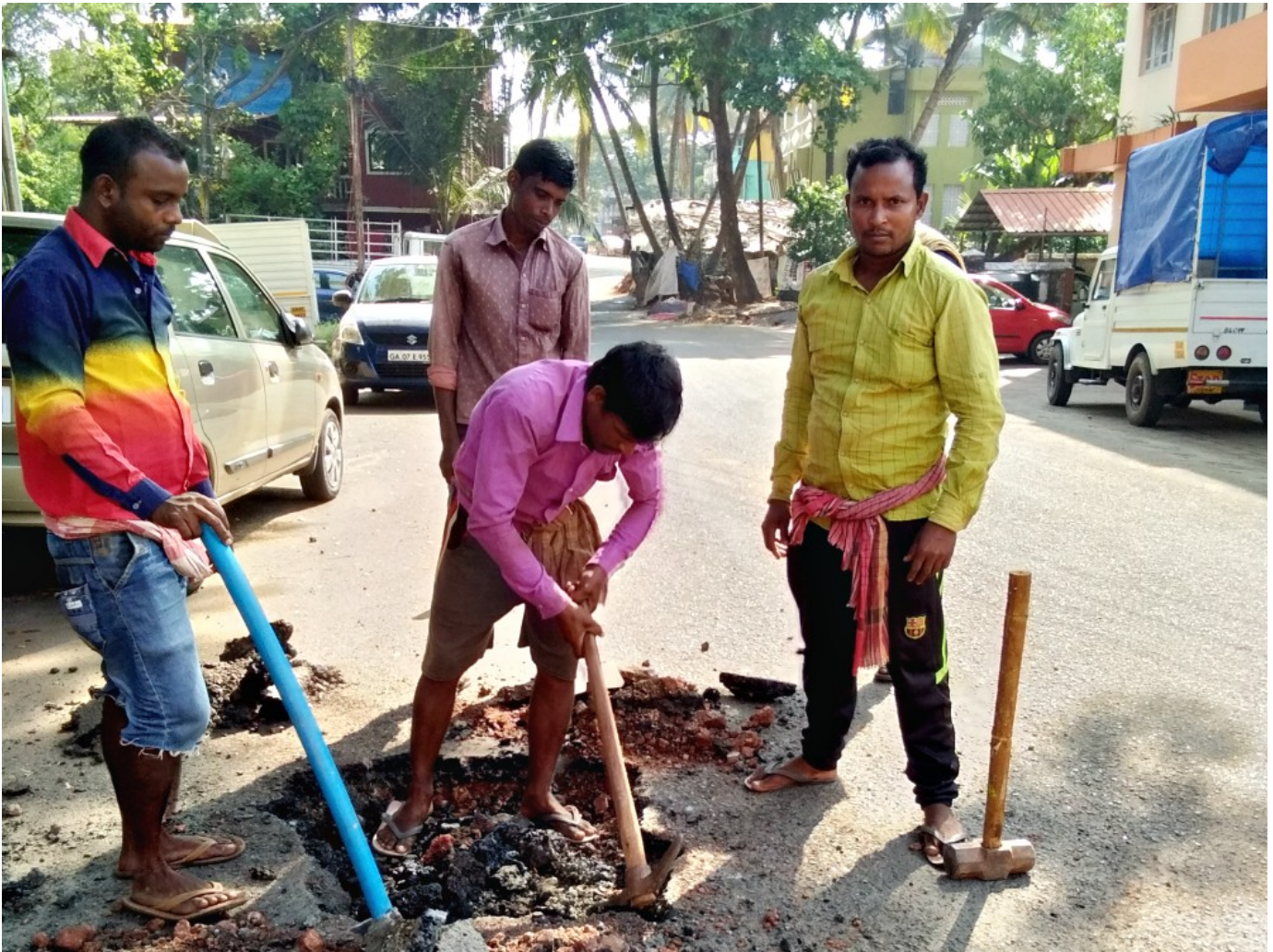
Migrant men repair a road in Mala, a village in Goa, western India. (Lissy Maruthanakuzhy)
