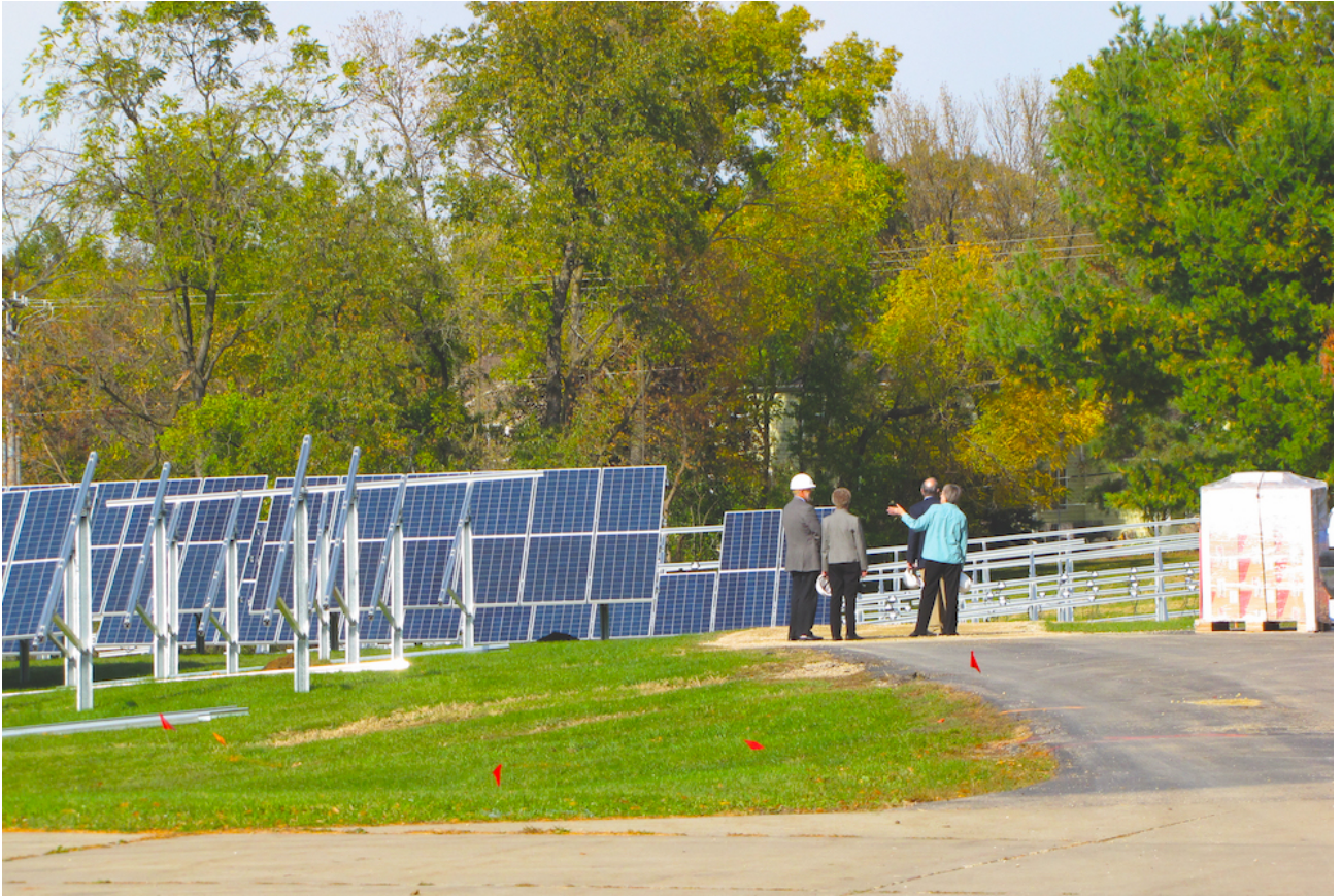
Touring the solar panel array in 2014, when they were about one year old on the property of the Franciscan Sisters of Rochester, Minnesota (Franciscan Sisters of Rochester, Minnesota)
